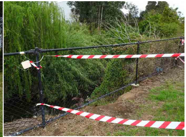
Erosion between sportsground and creek bank
