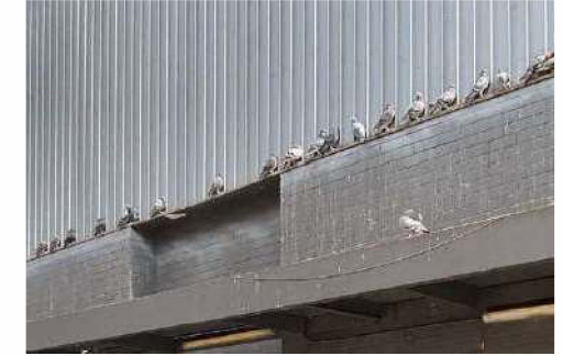
Pigeons roosting on facade paneling.
