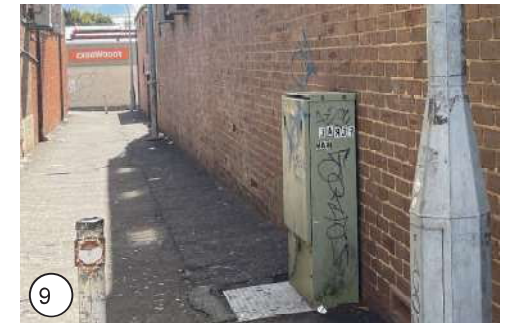
9 Graffiti tagging and general begrimed condition of Guildford Laneway
