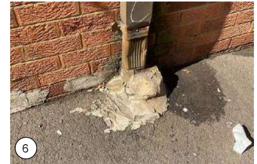
6 Condition of infrastructure in Guildford Laneway
