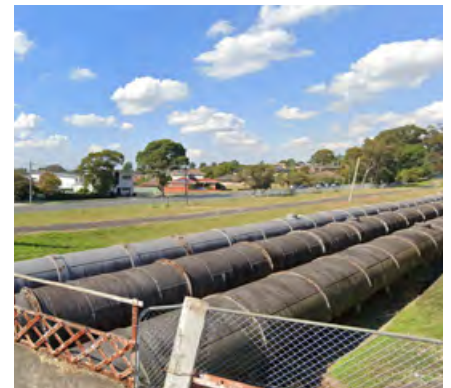
Figure 128 Exposed Pipelines (Source: Google Map)
