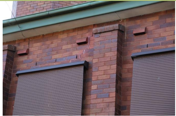
Detail of cracking to Church wall.
