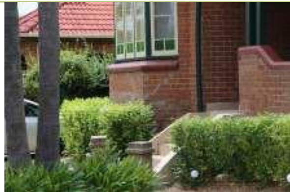
Detail of brickwork which has been poorly repointed.
