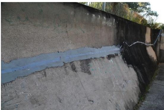
View to cracking of wall at Boothtown Aqueduct.
