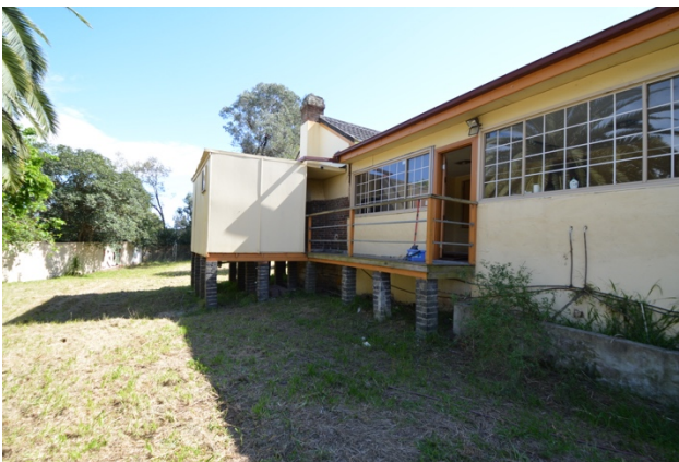
Figure 4.9 | Infill of the once-external space between the mirrored rear wings of The Wattles .
