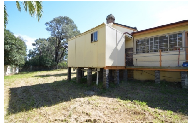
Figure 4.6 | SW corner showing accretions at the rear.
