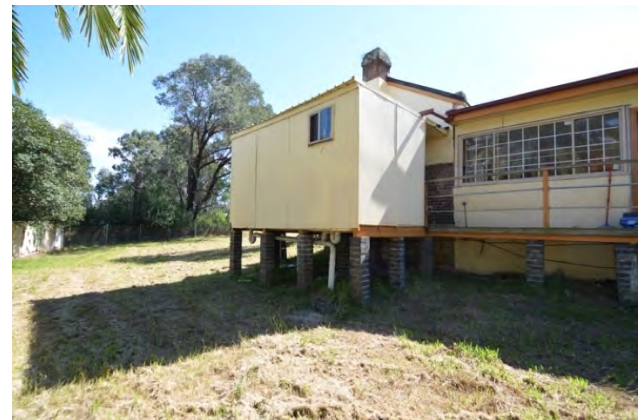
Figure 4.6 | SW corner showing accretions at the rear.
