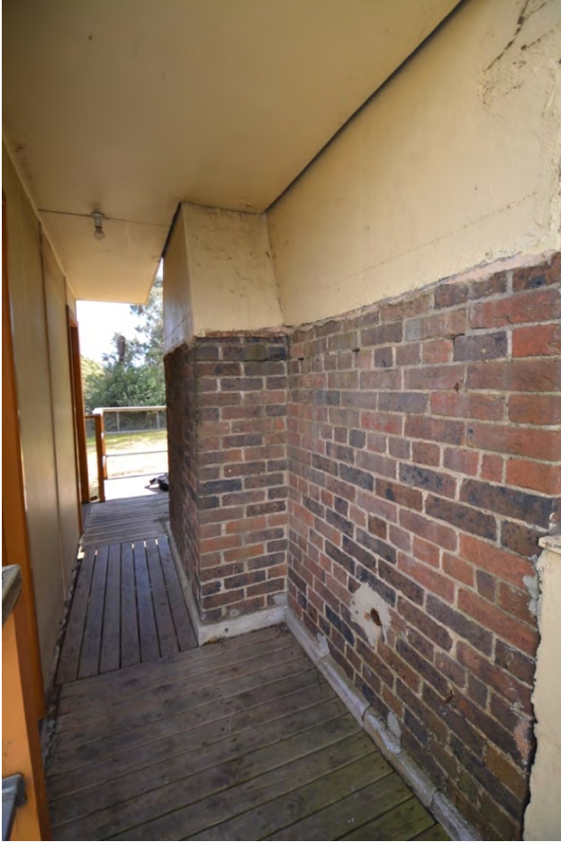
Figure 4.7 | SW side of the rear of The Wattles. Chimney breast and chimney extant.
