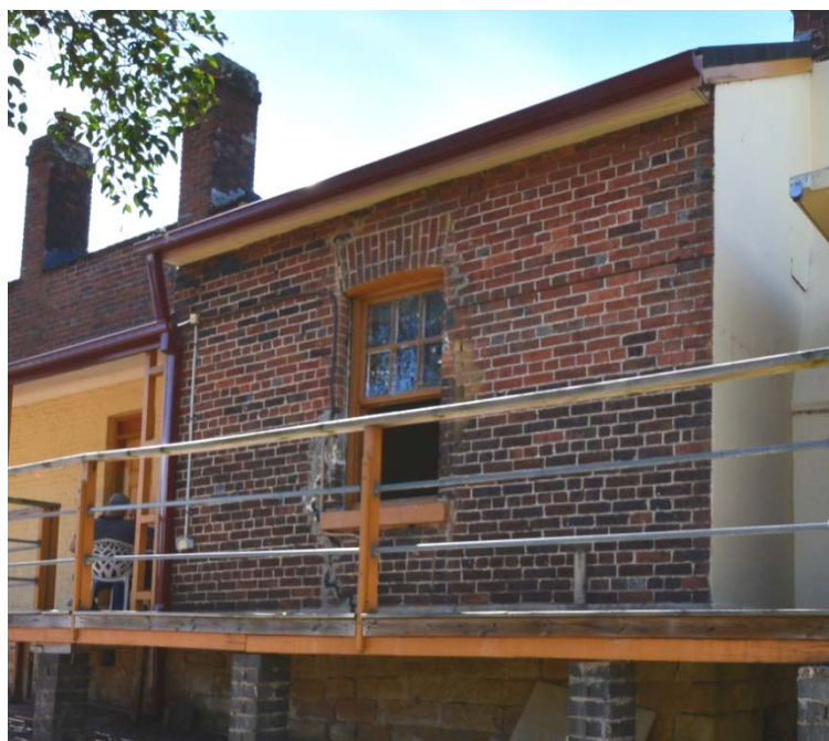
Figure 2.11 | Cracking in the western wall at the rear of the building has been an ongoing problem. Attempts to repair it in the past has been carried out crudely.
