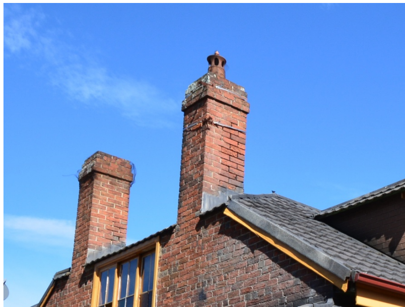
Figure 2.10 | Deteriorating brick pointing in the northern chimney on the eastern side of the house.
