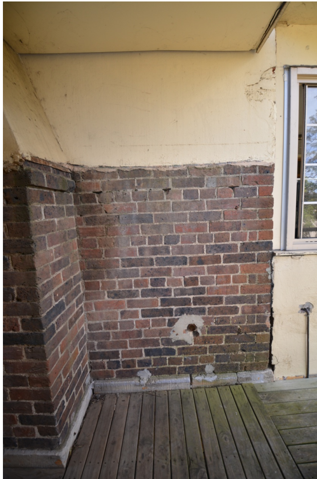
Figure 2.12 | Brickwork on the southern side of the southern wings (Rooms 6 and 7) requires repairs to mortar, replacement of new bricks where holes have been formed and careful removal of cement patching.
